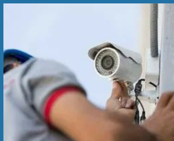
CCTV Camera Installation Service
